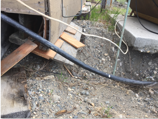
(Left) Hole opening up under the transmitter building. It doubled in size this year
