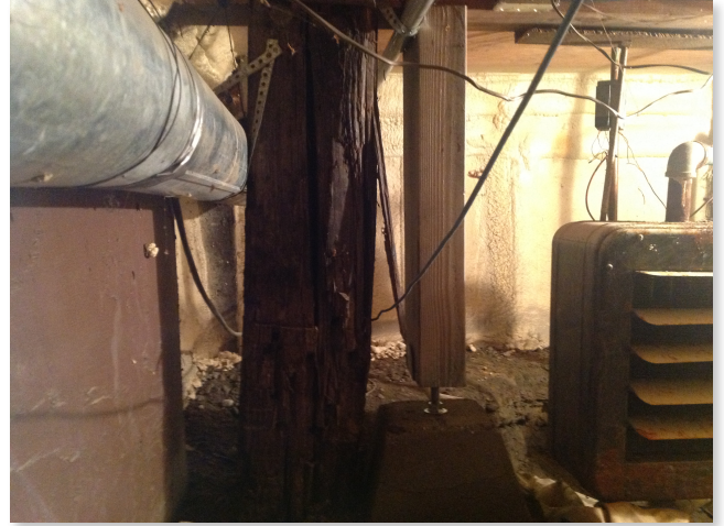
(Right) Rotting support posts under KIAM.
